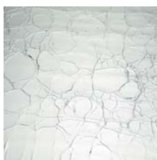
79 113 00 Ixx Cracked Ixx cracked
